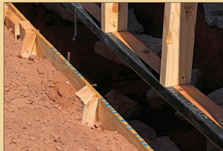
New base plates were wrapped with protective tape for a longer lifespan. Note the "J-bolt" concrete anchor hanging through the plate (upper left of photo).
