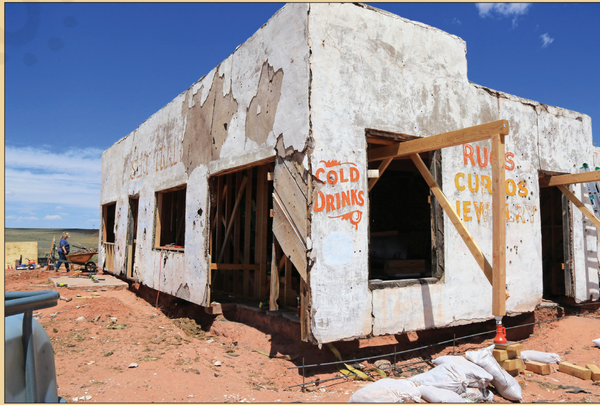
With shear walls on the inside and support beams extending through window and door openings, the trading post is fully levitated.
