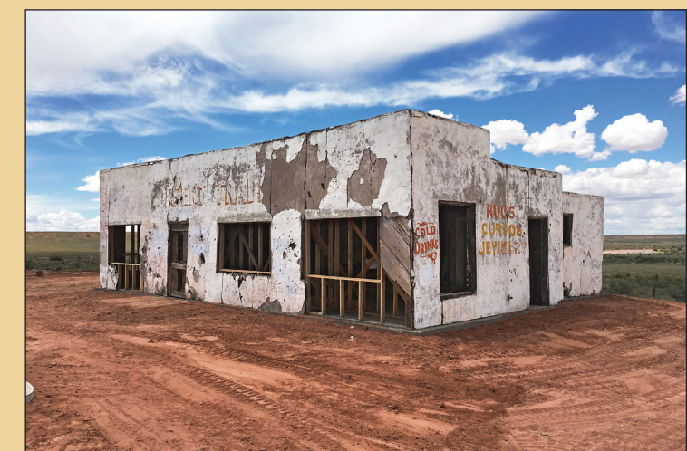
Backfilling and grading of the landscape brought the third phase to a close.
