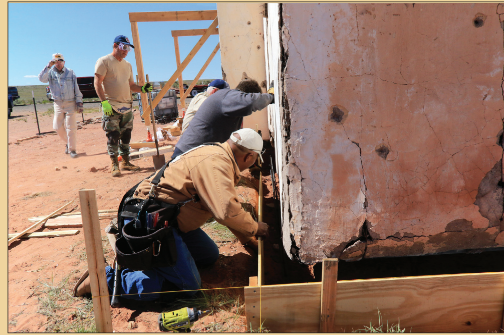
Concrete forms were set at the same height of the building's slab floor.
