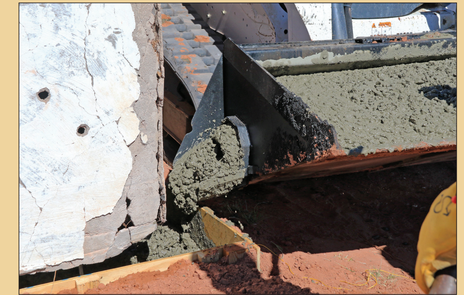
An inventive device created by a Co-Op member allowed for controlled dispensing of concrete into the footing.
